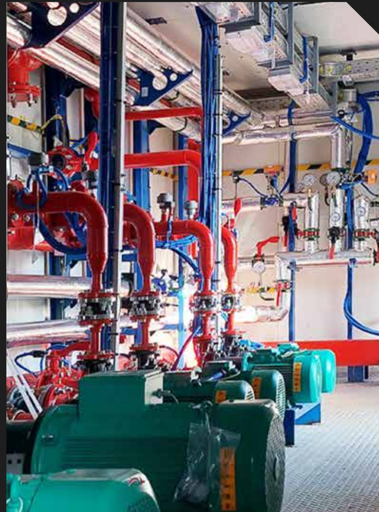
Block pumping station for a workers' settlement
