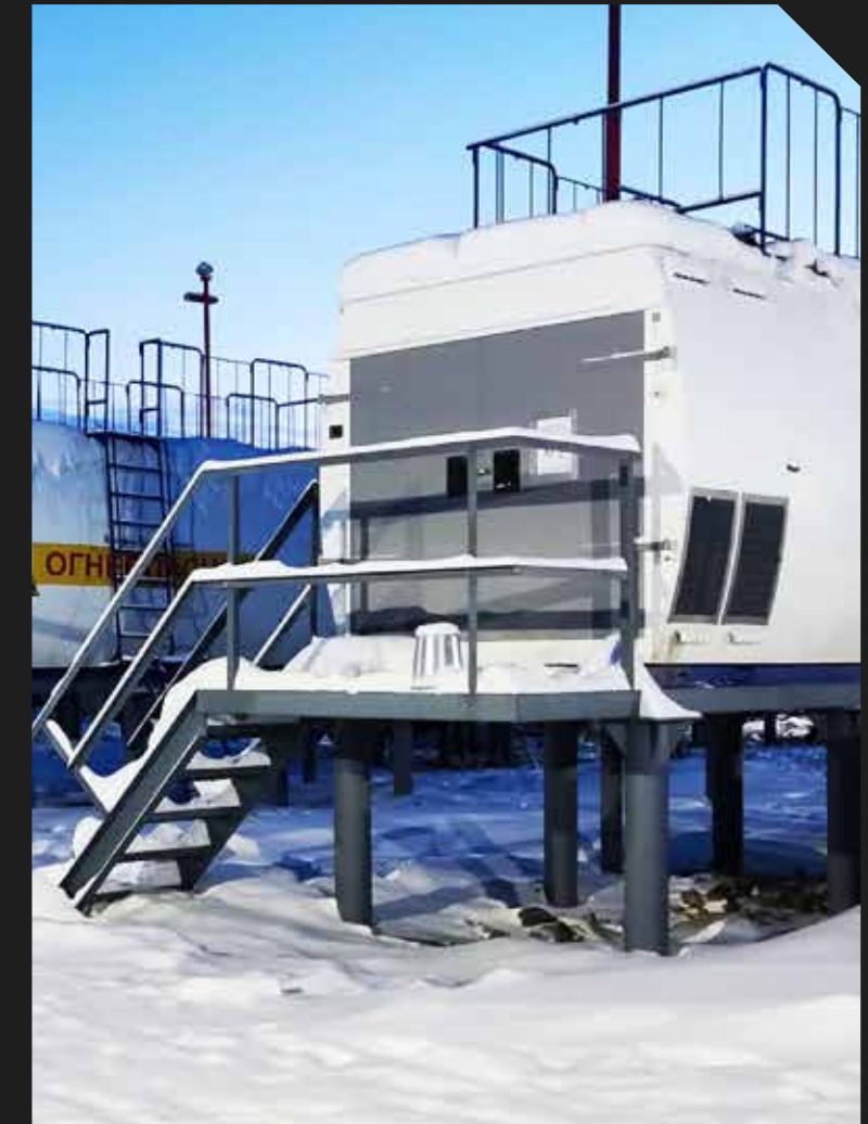
Fuel storage tanks
