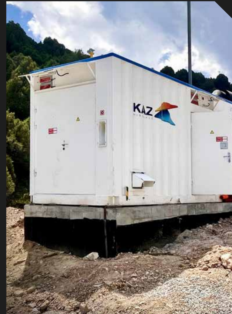
4.5 MW diesel power plant for underground mine in the Kyrgyz Republic
