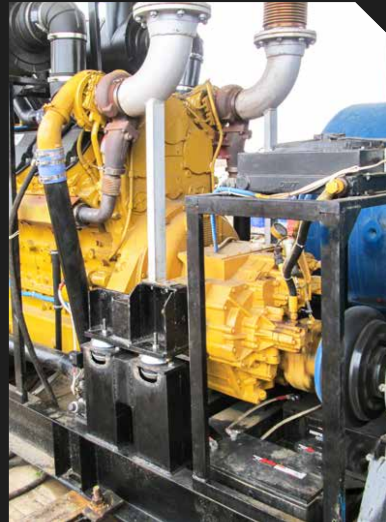
Well drilling pumps
