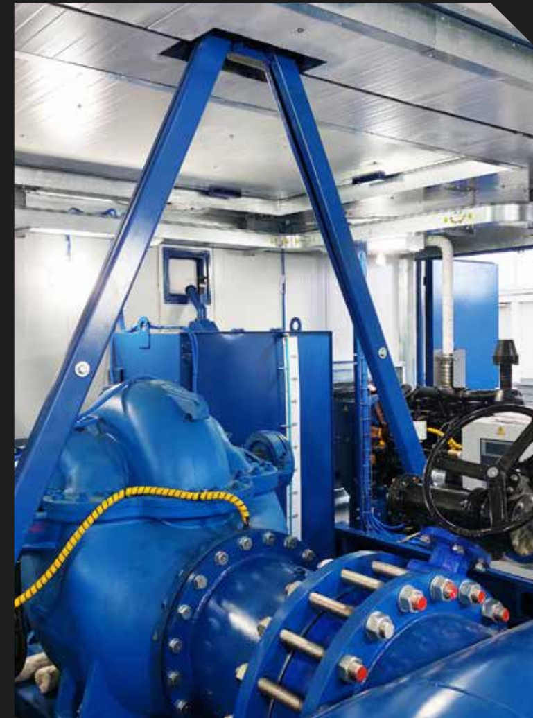
Diesel pump unit for gold ore field
