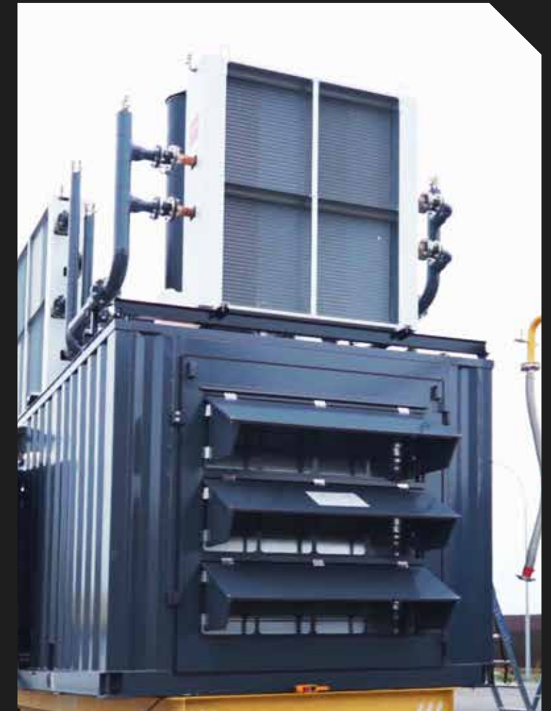
1 MW gas-fired power plant for glass factory
