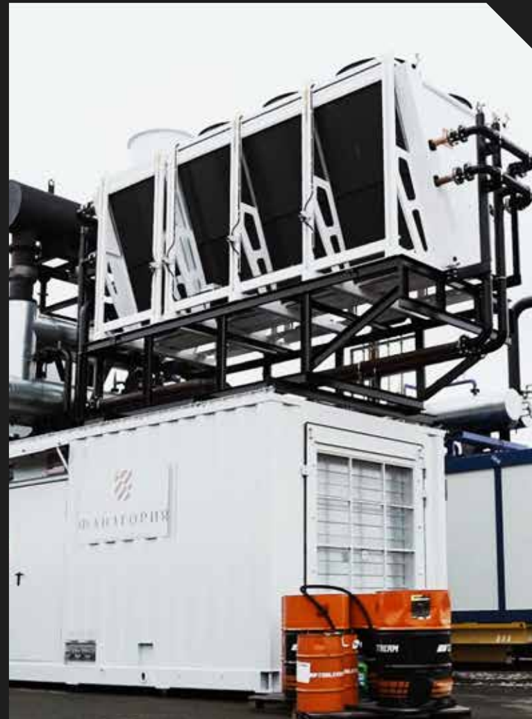
1 MW gas-fired power plant for Fanagoria winery
