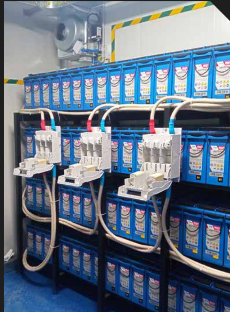
Uninterruptible power supply
